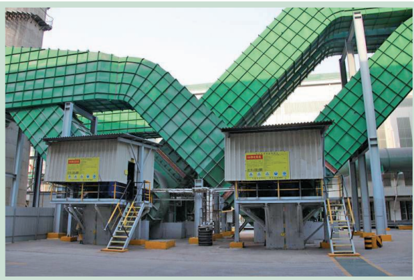
The transformed purifying draught fans
