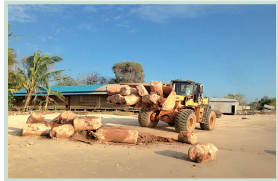
PT. Well Harvest Winning donating building materials to help the local’s repairing of the damaged coastline
