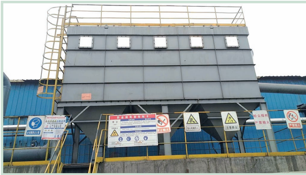
Modified explosion-proof dust collector
